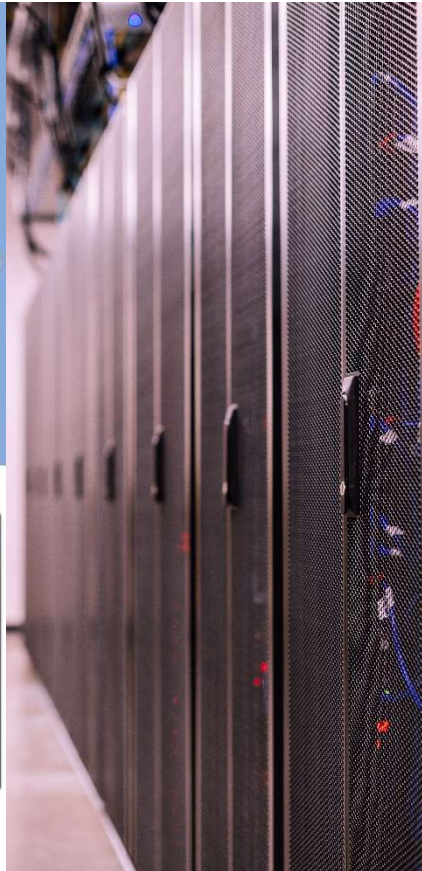
On-Site Data Server
